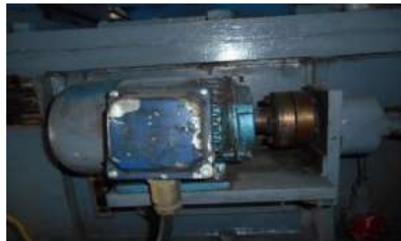
Gambar 1 Motor Pompa Gear Box APH
