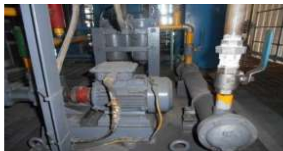
Gambar 2 Motor Pompa Thrust Oil Bearing
