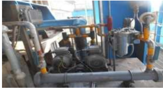
Gambar 3 Motor Pompa Radial Oil Bearing
